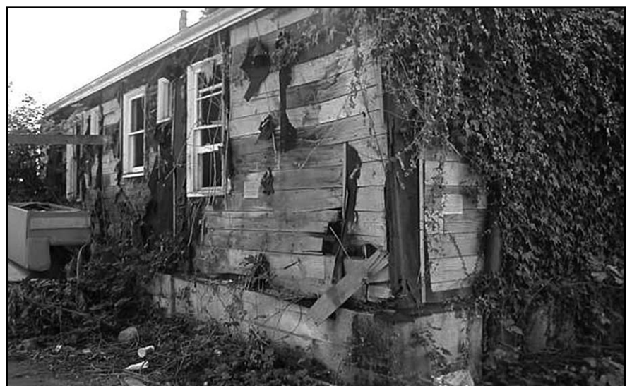
This dangerous building is termed an "attractive nuisance" and a fire hazard.
