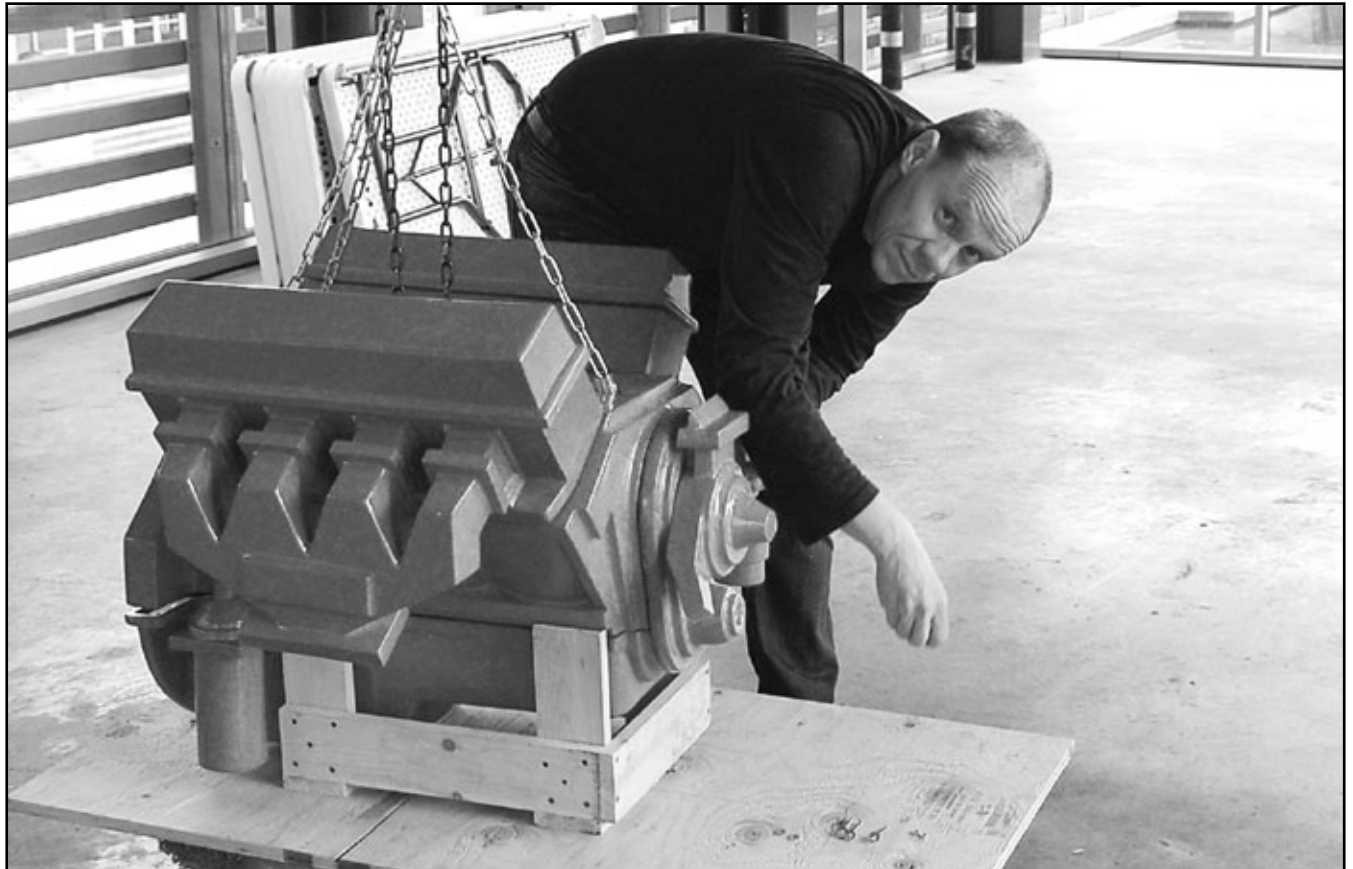
Artist David Packer of New York City installs "The Last of the V8s" in the Pavilion at City Hall. Five large, red, porcelain "engines" will hang from the ceiling of the building at the north end of the City Hall Plaza.
