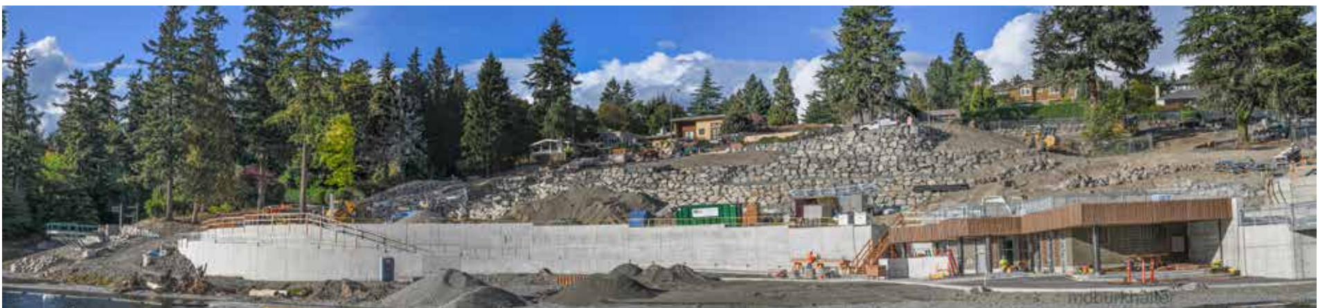
Panoramic view of the park under construction in September. Photo by Michael Burkhalter.
