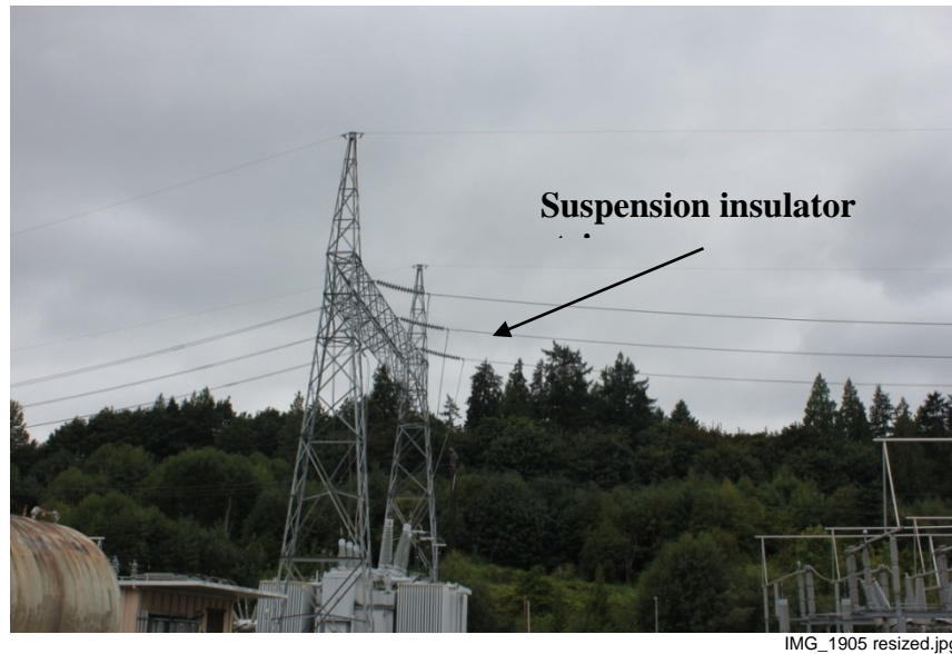
Figure 40. Suspension insulator string that might be vulnerable in case of a major earthquake
