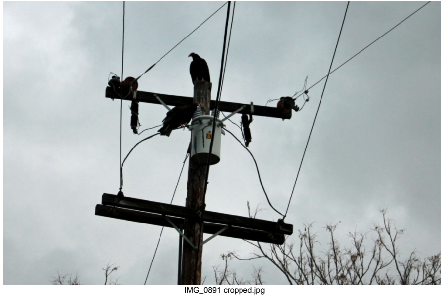
Figure 46. Turkey Buzzards Perched on Top of a 15 kV Distribution Pole and Transformer
