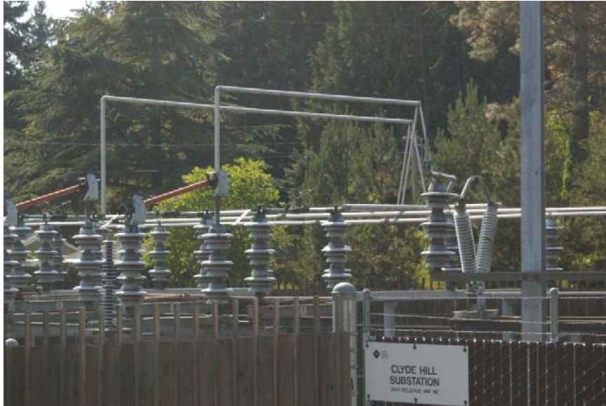
Figure 28. Clyde Hill Substation
