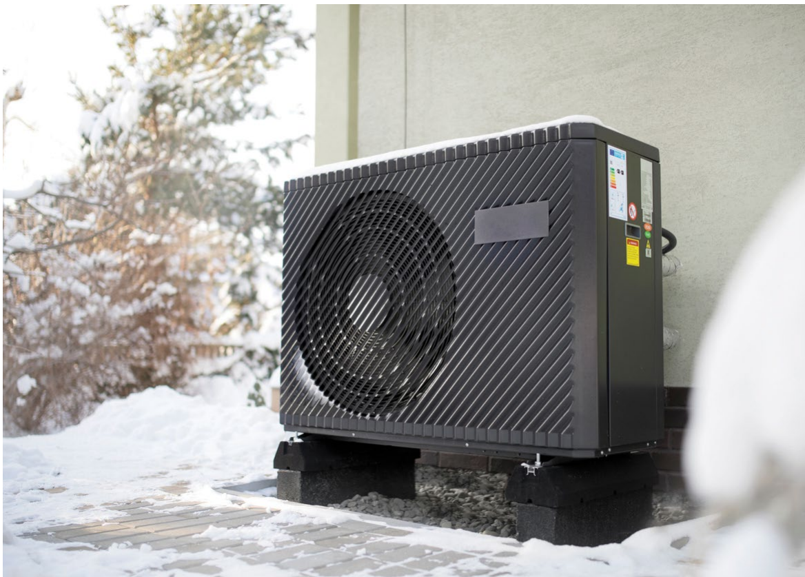
Heat pumps like this one provide energy-efficient heating and cooling.
