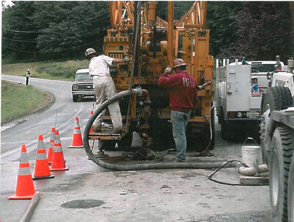
Photograph 5 - Close up of grout injection through drilled hole. Contractor ground monitoring "manometer" is visible attached to right-most outrigger.
