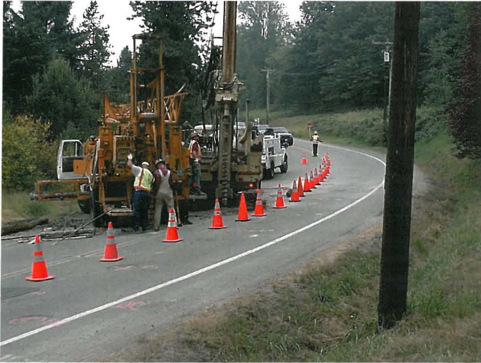
Photograph 3 - Looking north. Drilling in southbound lane with two drill rigs (Mobile B-61 in front of A-400).
