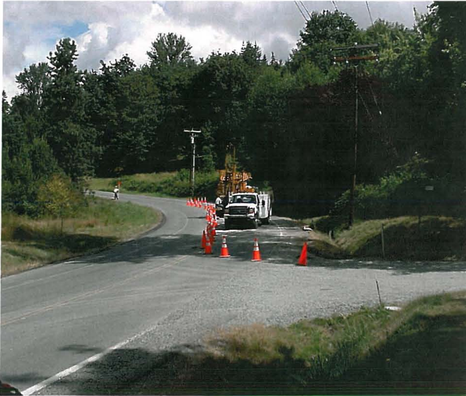
Photograph 1 - Overview of project site on Lakemont Boulevard, looking north. Entrance to Cougar Mountain Park in foreground.
