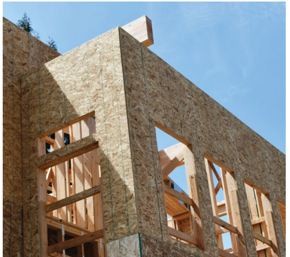
Your home improvement project can be a lot less ambitious than this addition and still need a permit.
