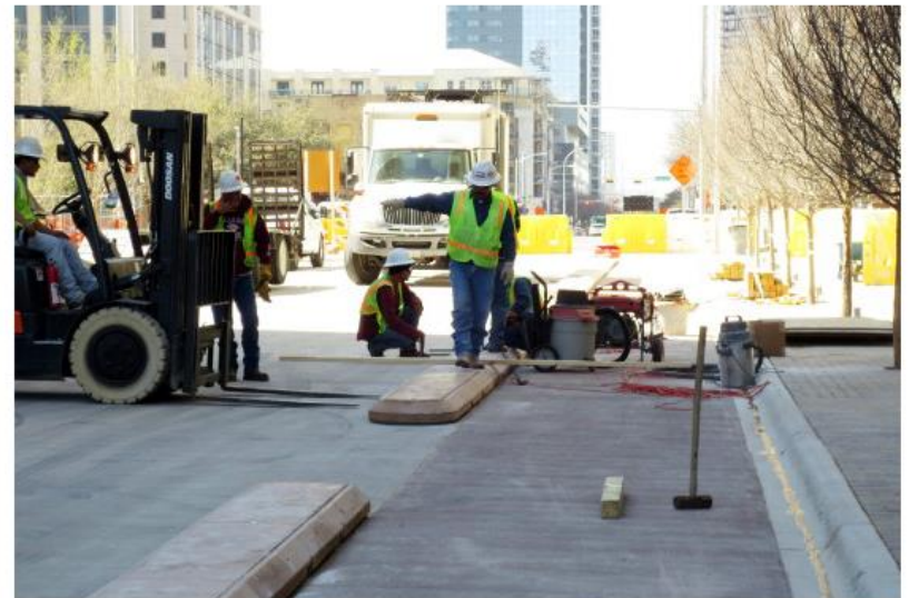
Austin workers set modular precast curbs in place on Third Street downtown.
