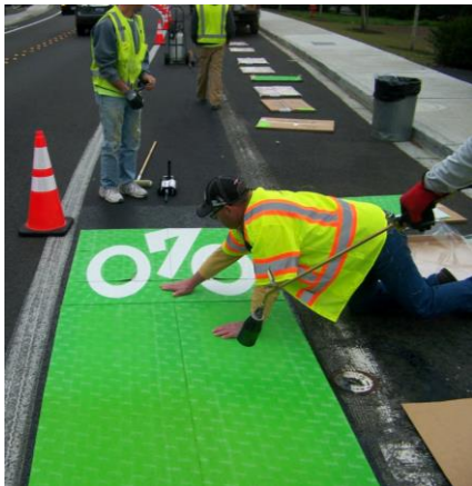
Installation of green bike lanes on SE Newport Way, near 150th Ave. SE.
